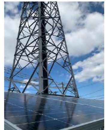
Sustainable Base Station
